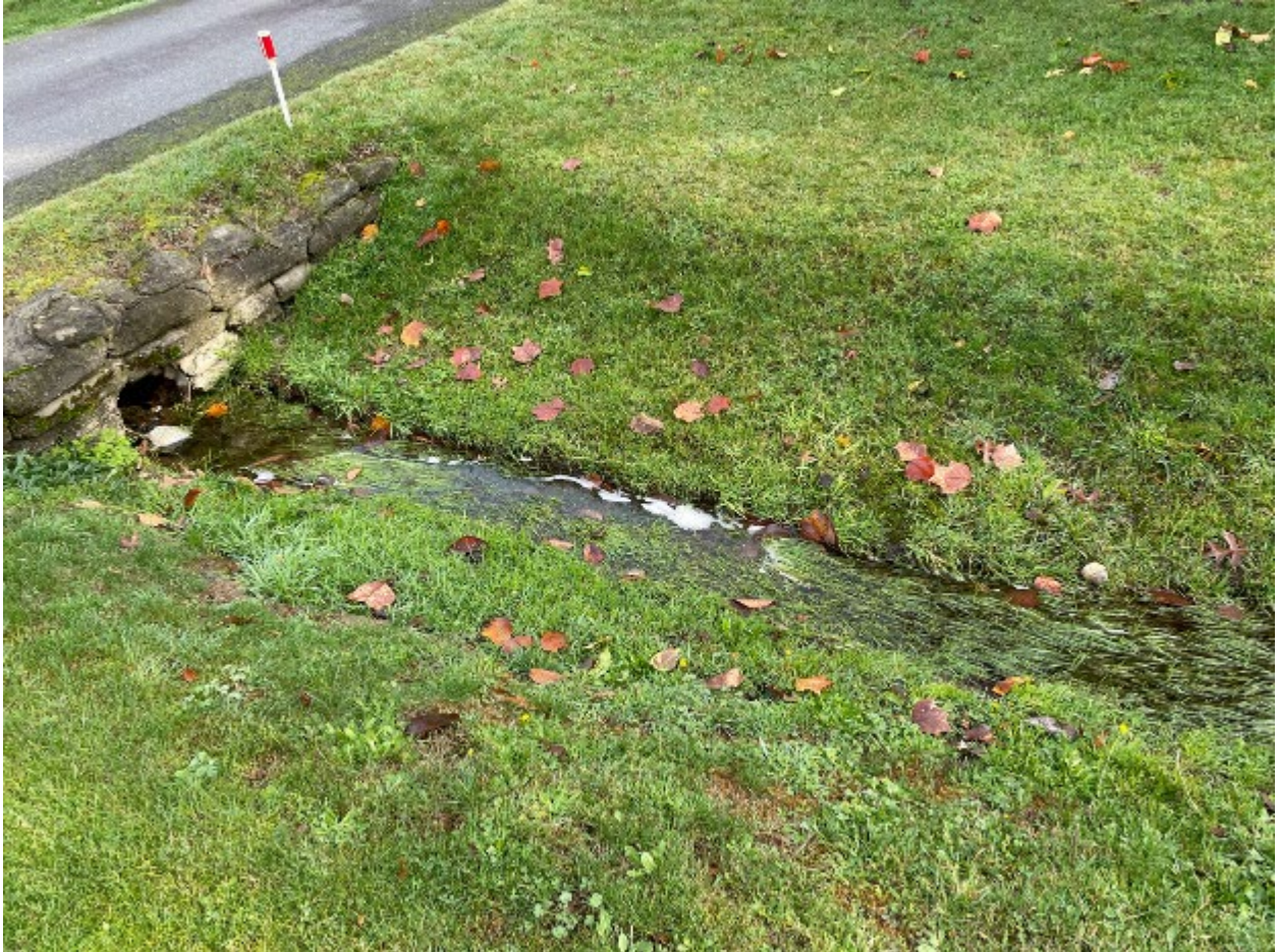
FIGURE 8: One of the storm drains that carries septic pollution towards Coles Bay. A build-up of pollutants that are causing a foamy substance at the surface is evident. Note the straight storm drain design that encourages a fast flow rate, without mitigation design such as rain garden or wetland. (Photo: Camille O'Sullivan)
